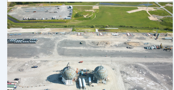
Ongoing construction of Plug Power's project at STAMP was highlighted by the spheres that will store the green hydrogen manufactured on-site using electrolysis.
