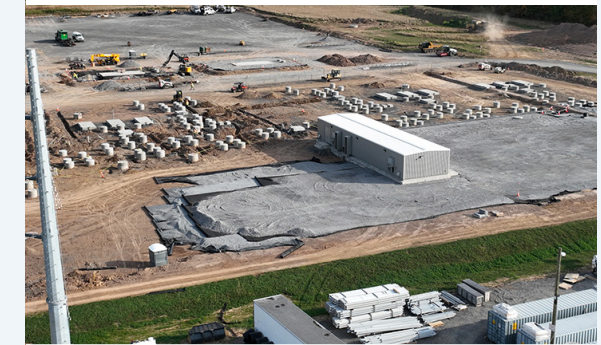
Construction of a 600-megawatt substation connects high-capacity power lines to a distribution system bring renewable-sourced electricity to companies at STAMP.
