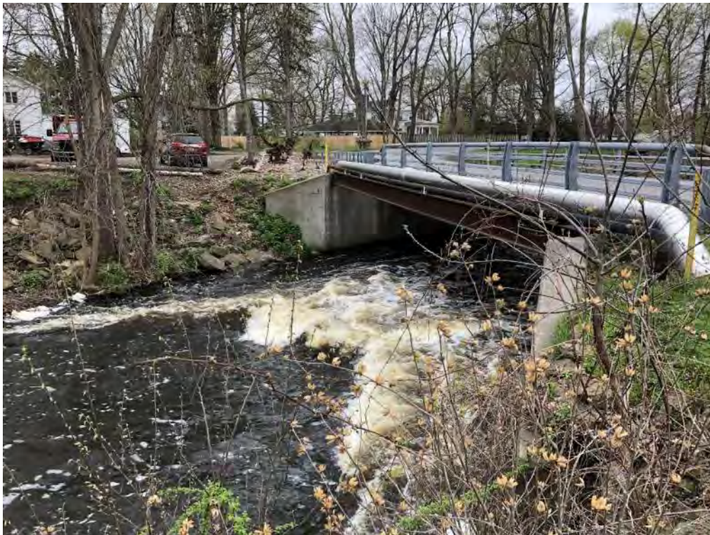
Photo 2: Looking downstream from right bank at Main Street bridge and upstream attached pipe bridge.
